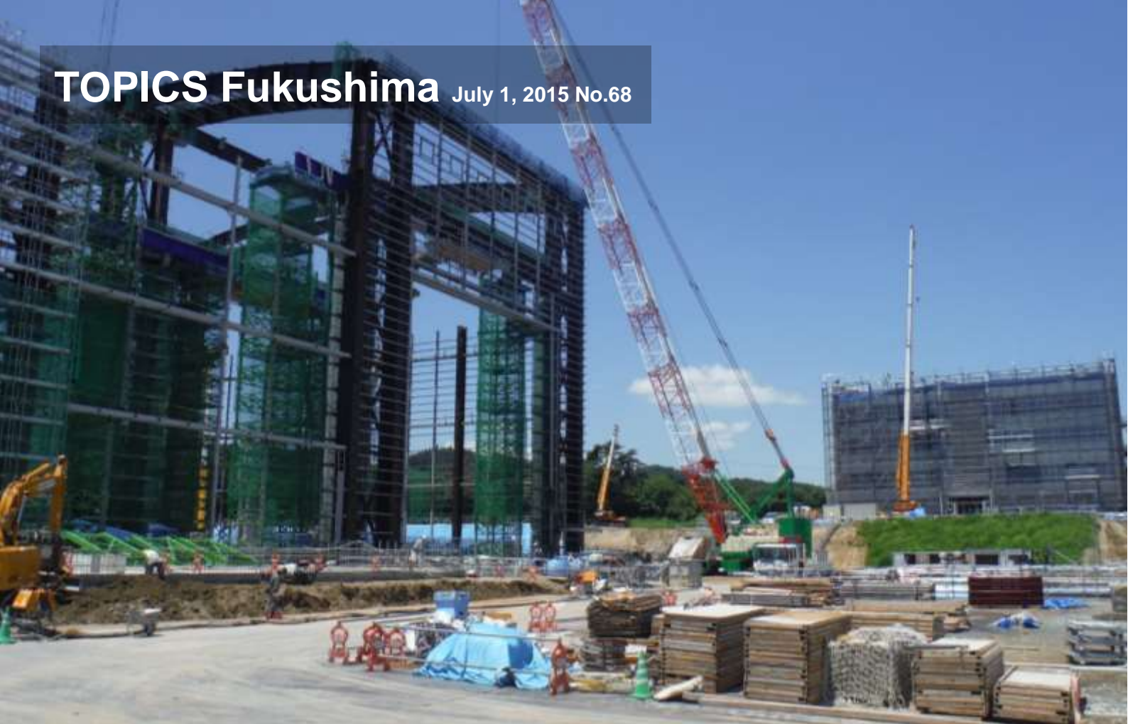
Construction of the Naraha Remote Technology Development Center. Research management building located far right, Demonstration test building front left. Taken with wide-angle lens
