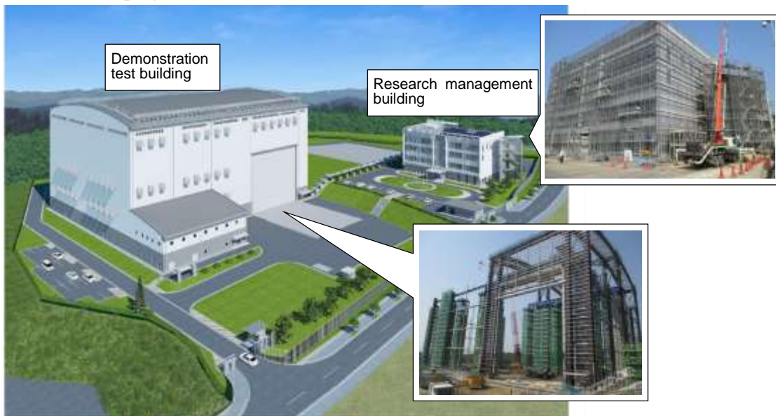
Fig. 2 Image of the completed Naraha Remote Technology Development Center, and construction in progress
