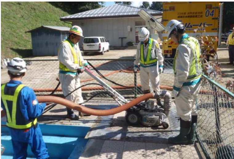
The photograph above shows decontamination work The photographs at the upper right and lower right show the pool side before and after decontamination
