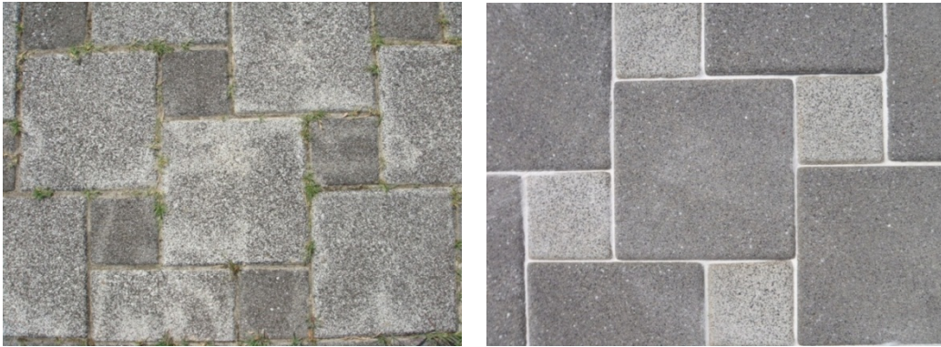
Fig. 3 Decontaminated place (upper pictures) and the surface of the pavement (lower pictures) of before and after decontamination. The left row is before decontamination, the right row is after decontamination. The old mortar joint sand was removed by decontamination, and white mortar joint sand was newly poured after decontamination.
